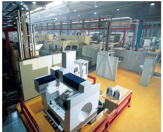
Example of Installation on Production Floor
